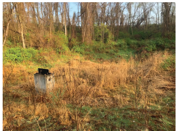
Excess Vegetation, Ponding Water Present, Outlet Structure Obstructed
